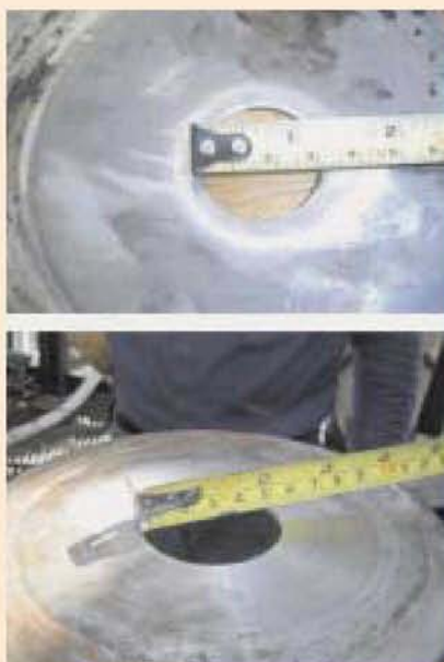
Figure 5. Dimensions of the orifice of the heavy liquor recirculation line from 1A concentrator to 1D concentrator, increased in April 2005
