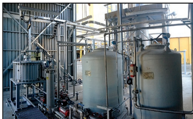
Figure 1. Ion exchange technology for chloride removal. Installation at Arauco Constitución mill. Left: SSU (Salt Separation Unit) - Right: process tanks
