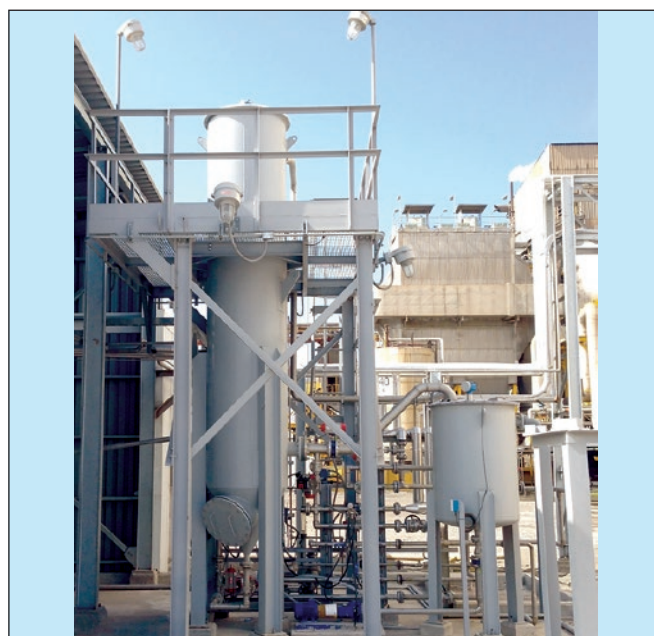
Figure 5. Installation at Arauco Constitución mill Left: pulse filter - Right: break tank
