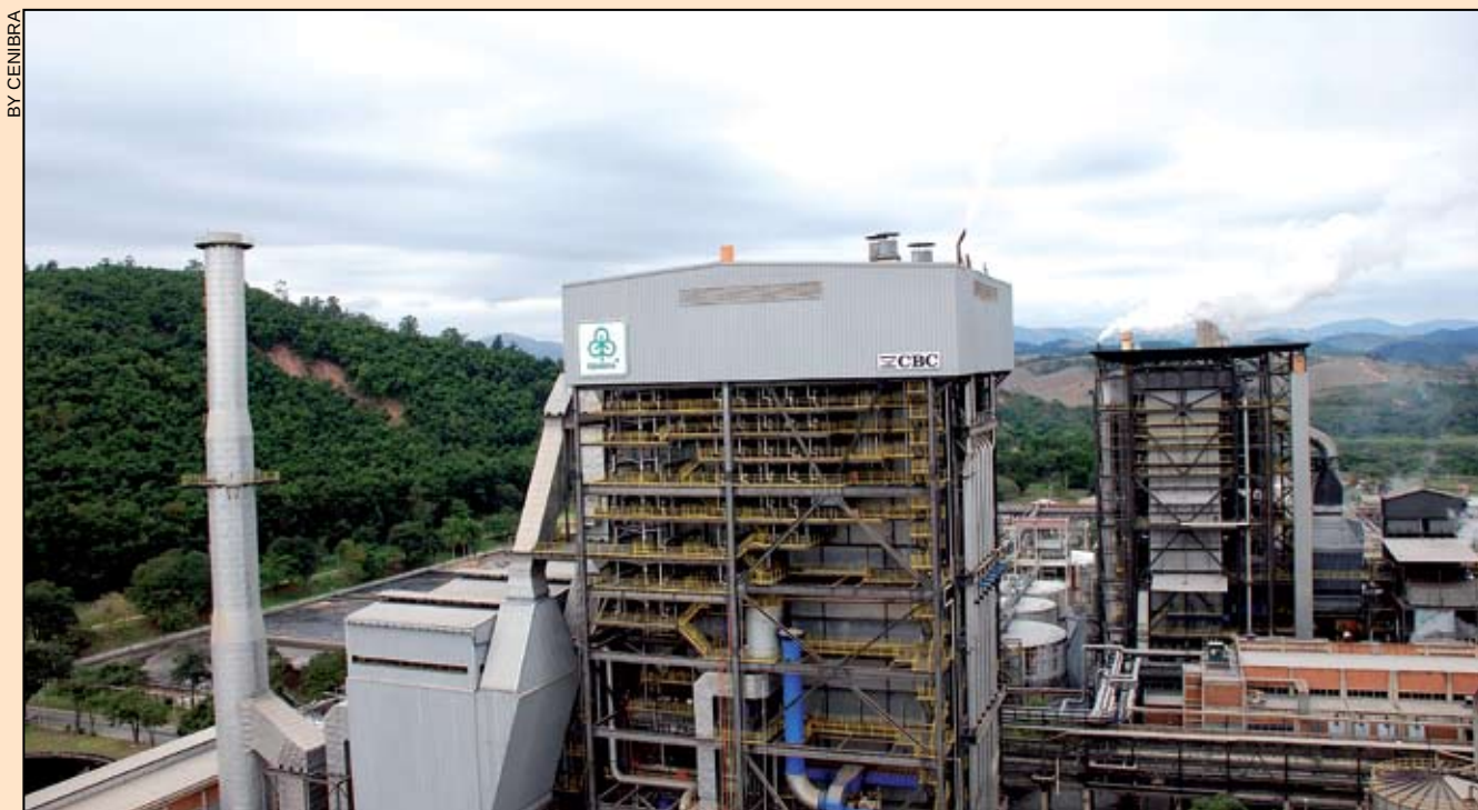
Nowadays boilers are five times bigger than the old ones
