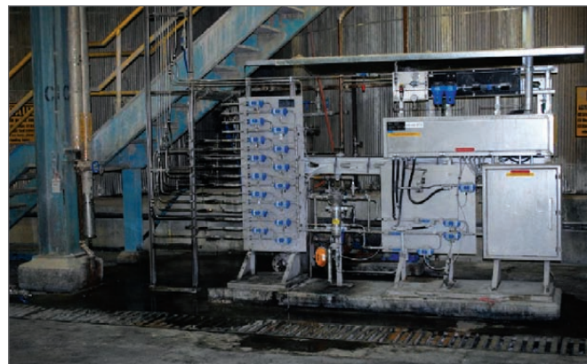
Figure 2. FT-NIR liquor analyzer sampling station showing sampling tree and transmission cell
